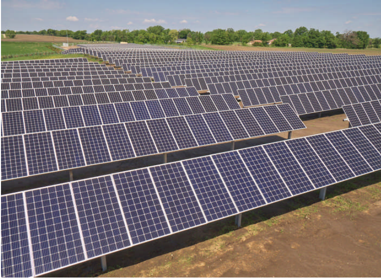
Minnesota Municipal Power Agency's 7 MW Buffalo Solar Buffalo, MN
