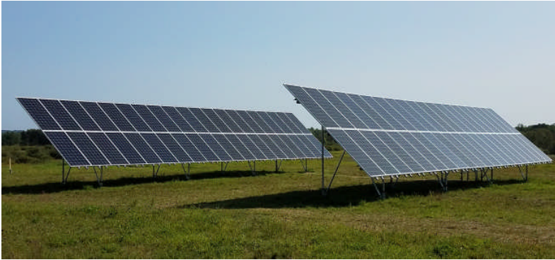
Detroit Lakes Public Utility's 29.3 kW Select Solar Community Solar Garden Detroit Lakes, MN
